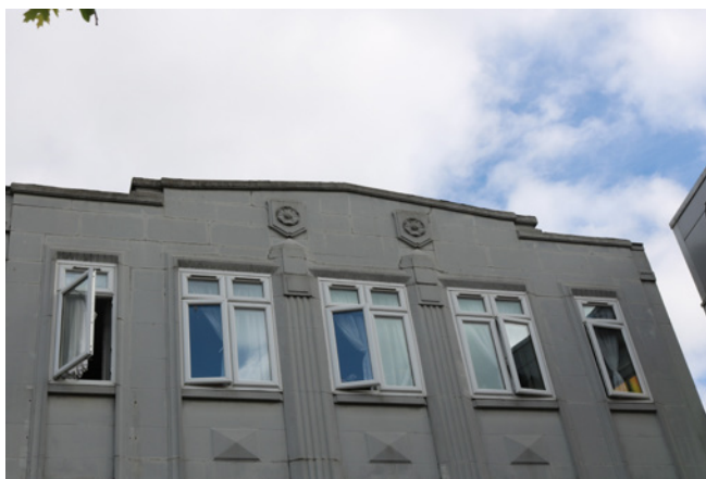
Insensitive uPVC window replacement, South Street
