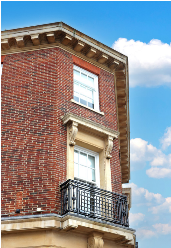
Detail of timber casement windows and stone detailing within the corner façade of the Lloyds building.
