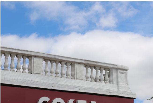
Detail of the balustrade No.83 South Street, part of a longer range that features at the southern perimeter of the conservation area.
