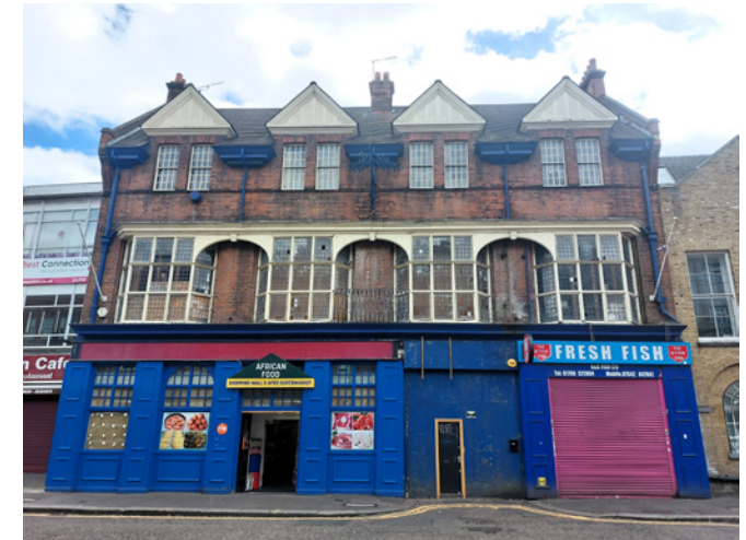
Brickwork and glazing damage to locally-listed White Hart façade on the High Street
