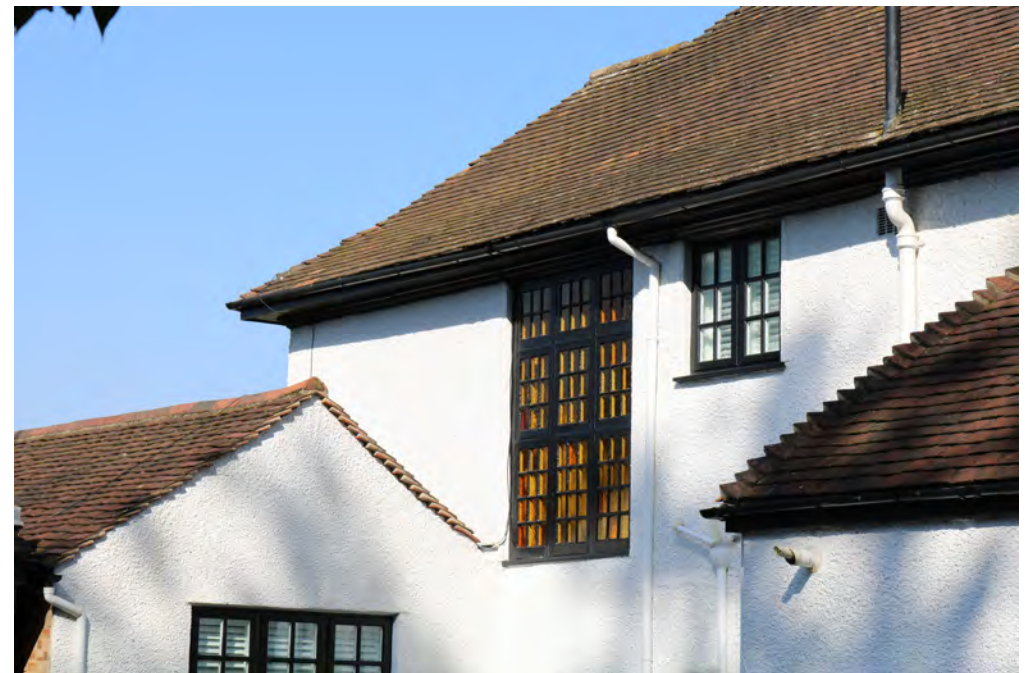
Detail of window, roof and façade materials used on Reed Pond Walk
