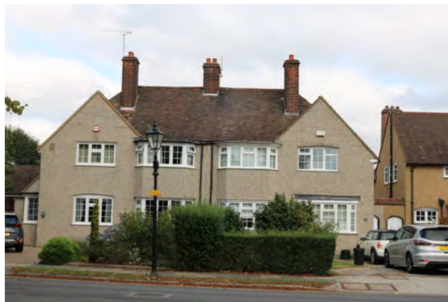
Insensitive window replacement, Balgore Crescent
