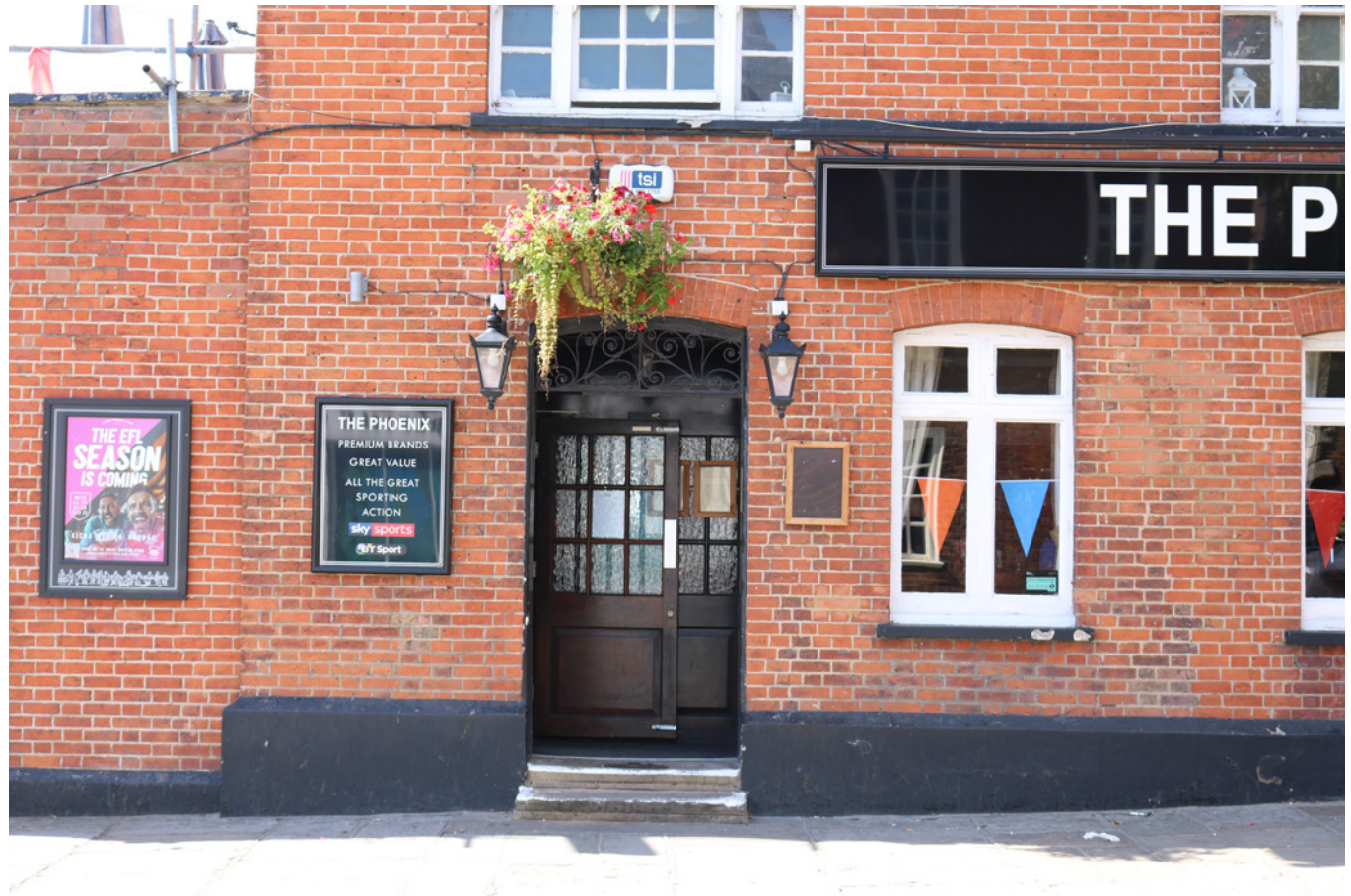
Surface-mounted services & conduit detract from façades
