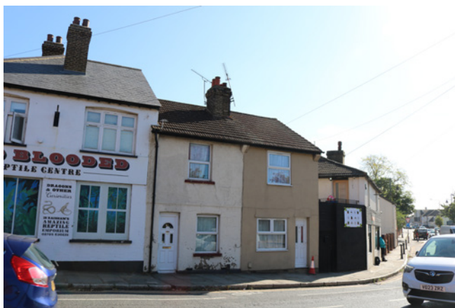
Render damage, Broadway
