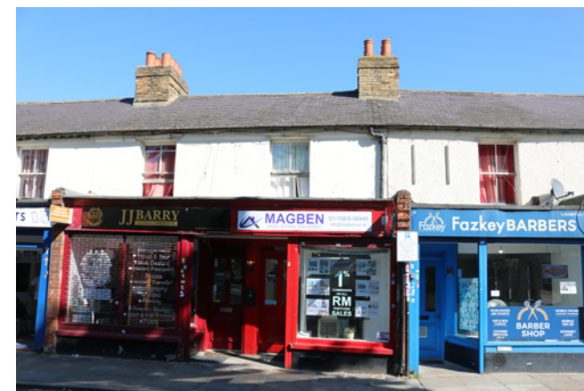
Some conservation area shopfronts comprise poor detailing and modern accretions
